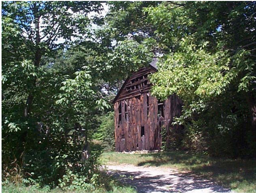
Hunt/Hosmer Barn, 320 Lowell Road. Probably 18th Century. Barrett Farm Historic District. One of the few remaining early “English” barns in Concord, it may be one of Concord’s oldest outbuildings.
